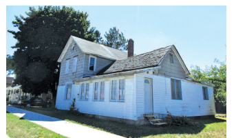
The Boyne City commission has officially agreed that this house at 204 S. East Street at the corner of Ray Street in Boyne City is "dangerous" and should be demolished. Father and son property owners Daniel and David Chapp are expected to take court action to stop the process so they can move forward with their plans to fix the structure.
